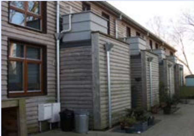
FIGURE 25: HOME RAINWATER CAPTURE SYSTEMS
